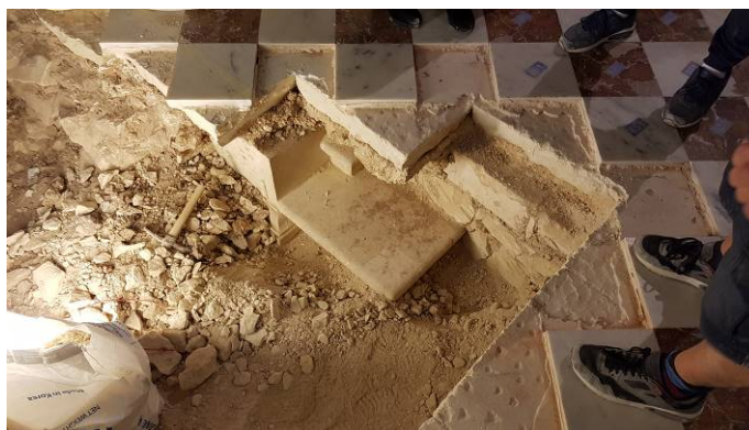
Figures 22a and 22b: Beautiful details (old steps and a lower 'original' floor finish) uncovered, thereby shedding light on the changes/ development of the Main Altar.
