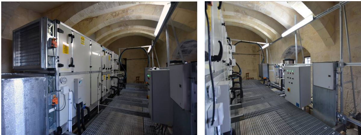
Figures 6a and 6b: The 'North Prison' fully equipped with the plant and equipment which is completely independent of the existing masonry fabric
