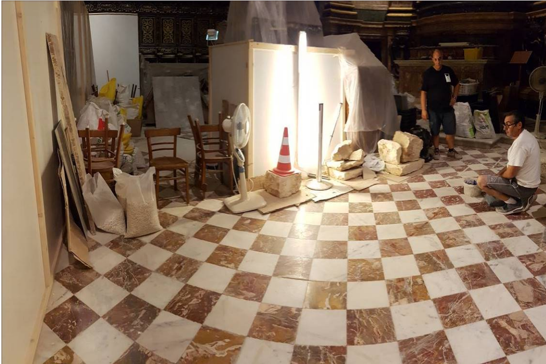
Figure 19: All the tiles were reinstated once the duct work was all installed and tested beneath the Main Altar
