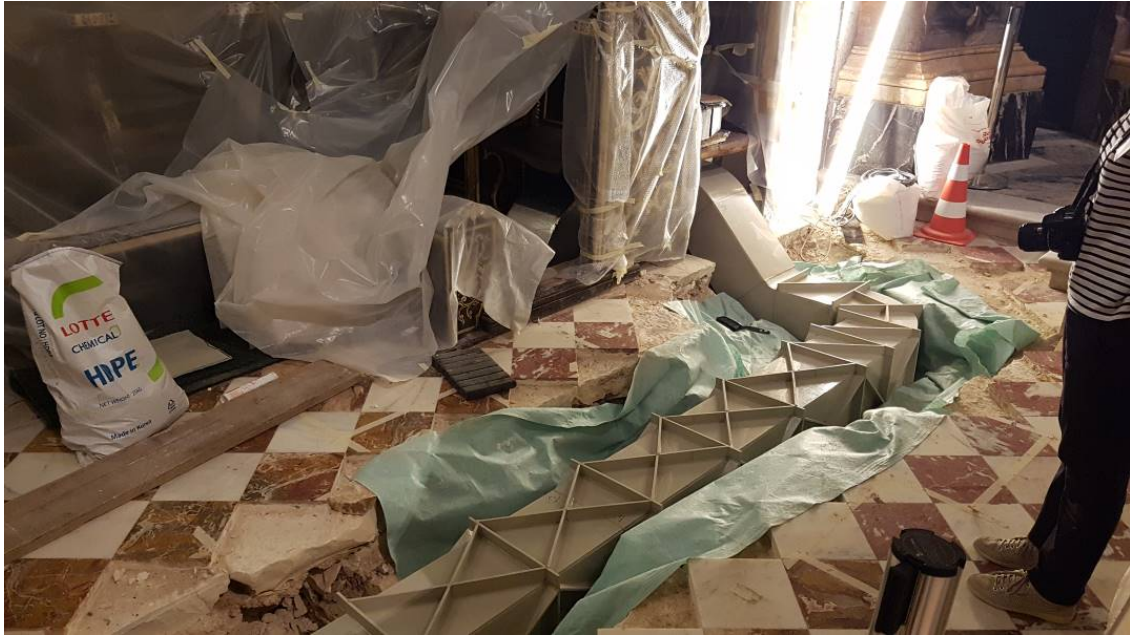
Figure 17: Reinforced and strengthened duct inserted within the space available with underlying geotextile.
